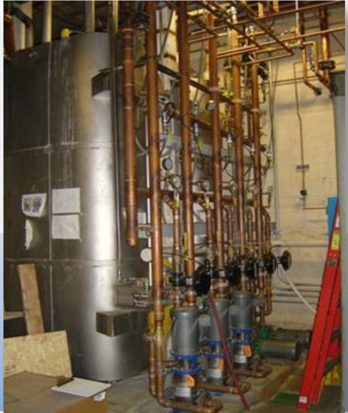
Steam Boiler System
