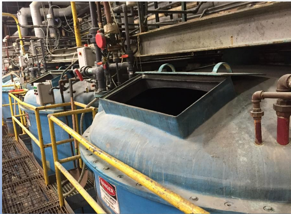
Existing reactor area
