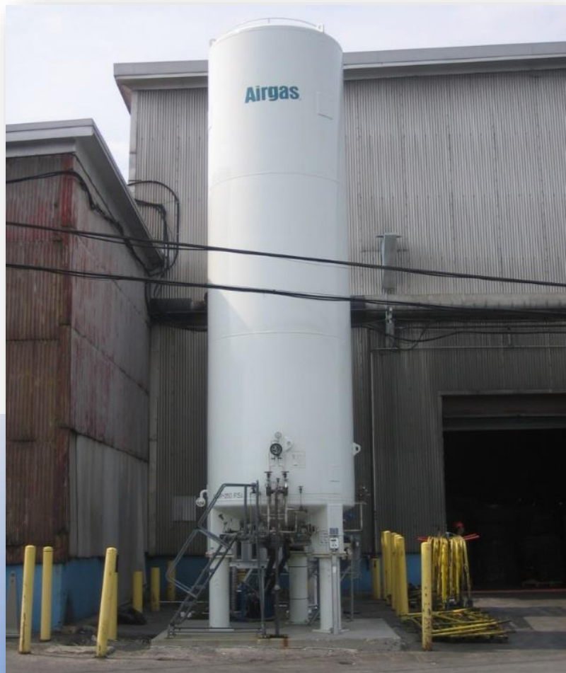
New liquid nitrogen tank
