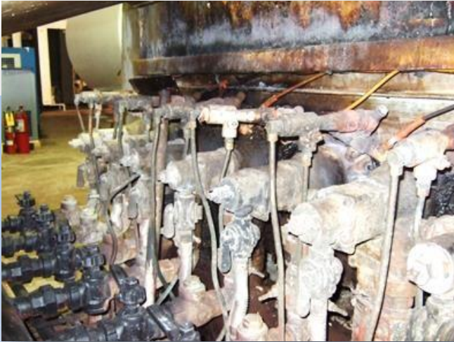
Previous burner system to be replaced.
