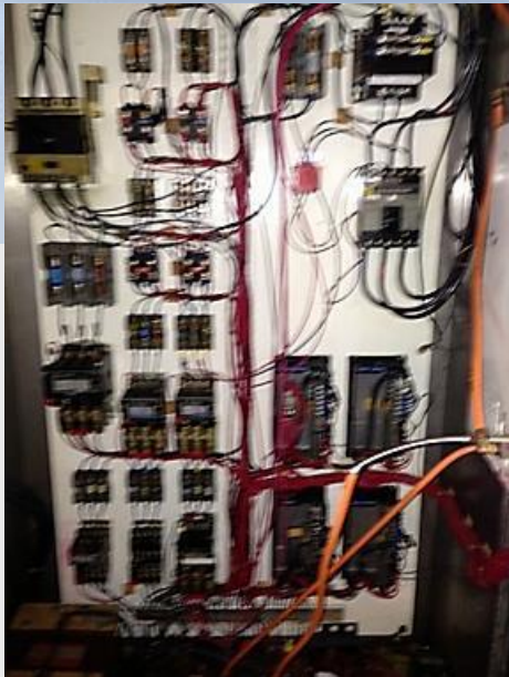
Old control panel to be replaced.
