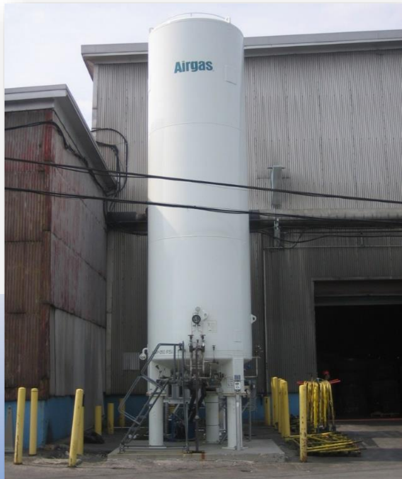
New liquid nitrogen tank
