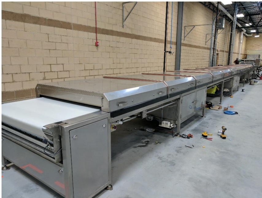
New cooling tunnel
